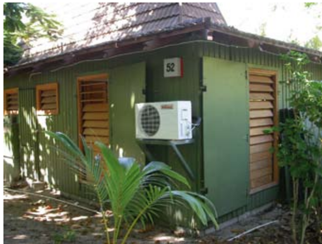
Figure 12.4 Air conditioning unit outside a tourist bungalow in Fiji *
