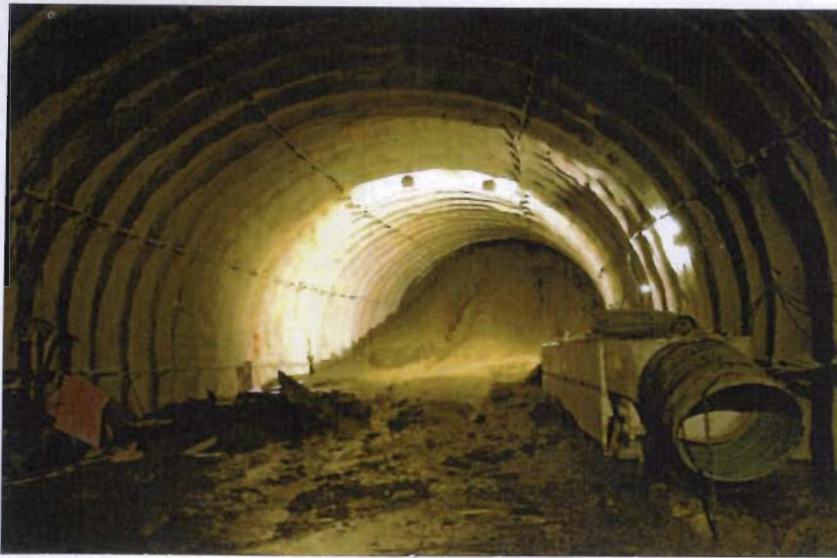
Left: View inside the collapsed Saint-Laurent tunnel
