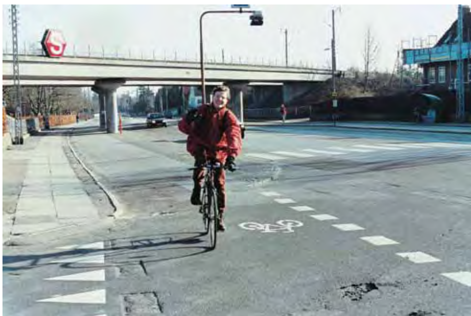
Potholes distract cyclists from traffic.
