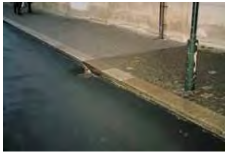
Be careful with drainage construction. The hole here around the grate is much too deep.
